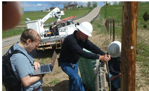
Figure 48 - Cablelabs Engineer Making a TDR Measurement in the Field (the SDR Is in His Backpack)
